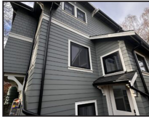
#11 - Green Lake Deep Energy Retrofit Carlisle Classic Homes 102 NE 64th St, Seattle, WA 98115
