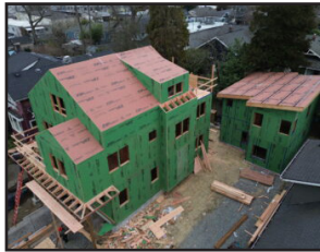
#10 - Phinney Ridge SFR + DADU Targa Homes + Pivot Windows 131 N 75th St, Seattle, WA 98103
